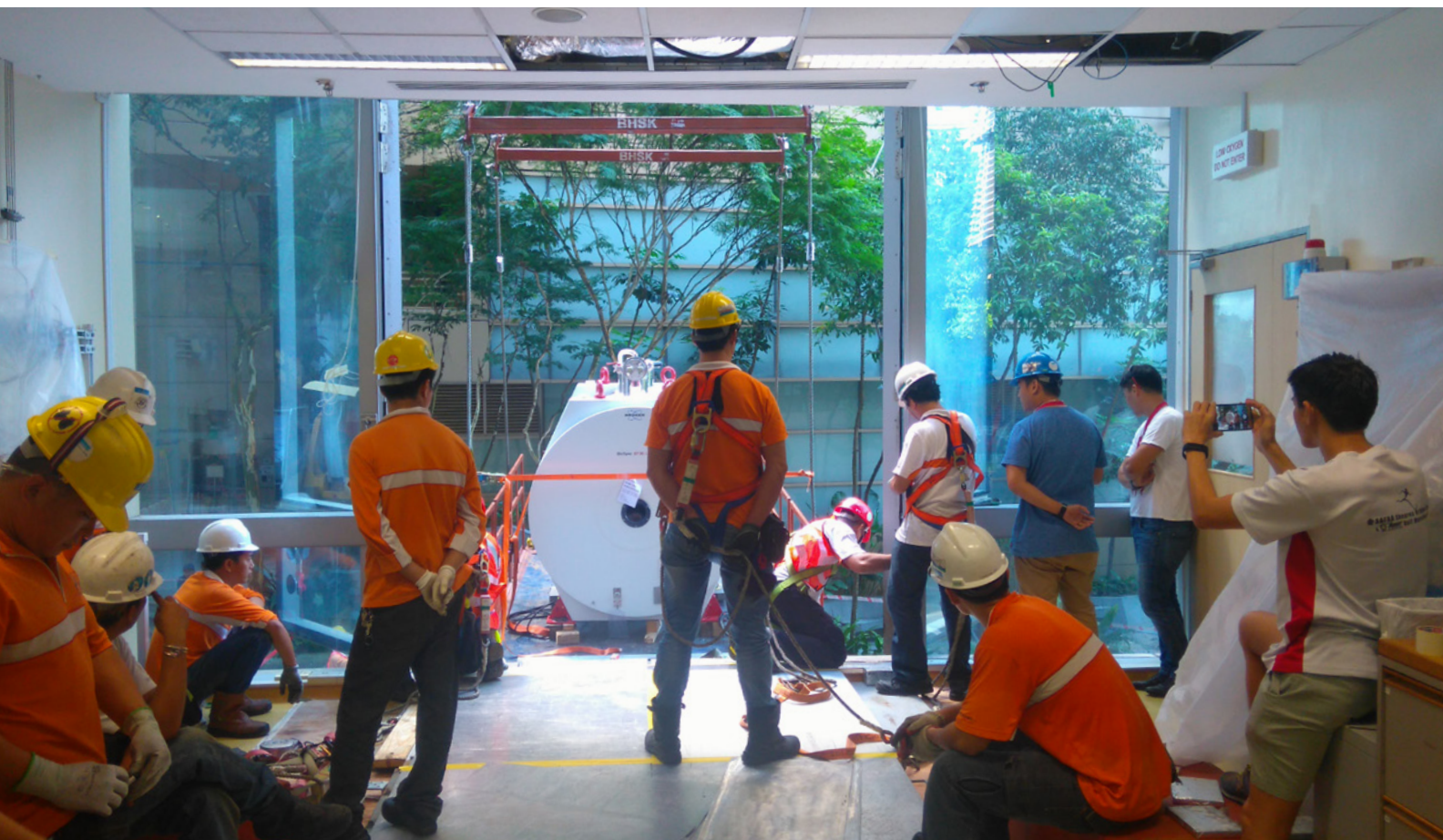
A 9.4T scanner, installed around 2013.
